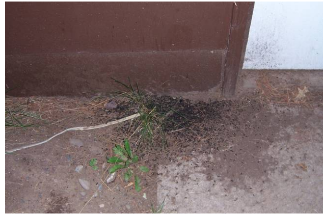
Bat guano in front of garage
